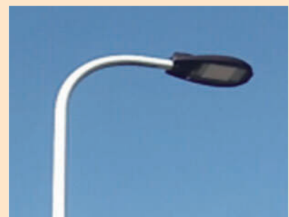
LED 街路照明灯
